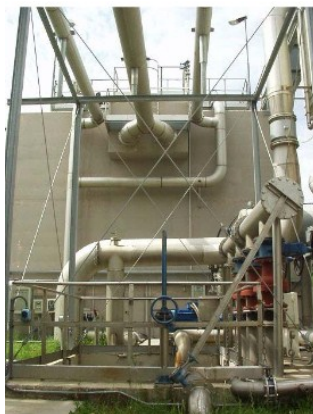
Figure 3 - Wastewater treatment plant in 1 st Macrolotto
